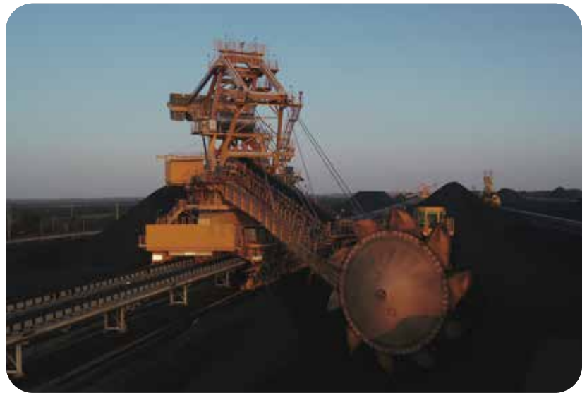
Port Waratah Coal Services, one of four major coal export terminals that use MRA's Stockyard Management System based on Rockwell Automation technology.
